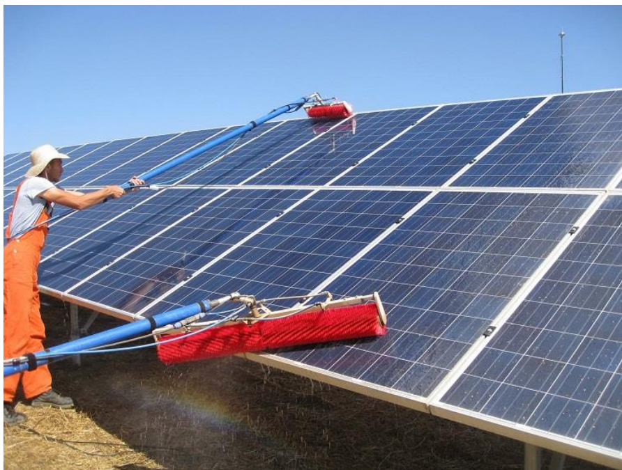
Figure 1.6.1: Labors manually clean the solar panels
